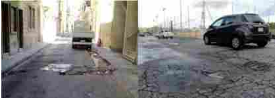
Figure 1 Potholes and cracks in roads observed in Sliema (left) and Sliema (right) of Malta
